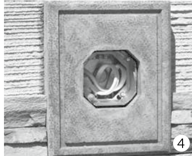
4 Complete placement of Modulo Stone veneer or other exterior material around Electrical Box Stone.
